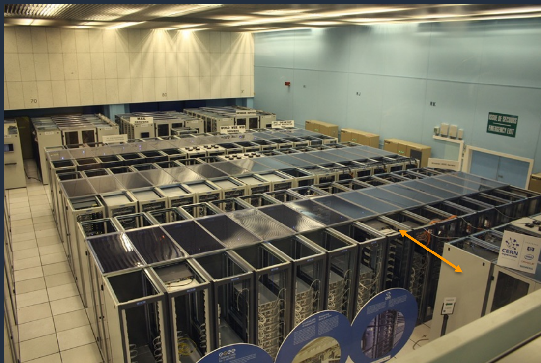
Traditional Telecom infrastructure exchange center
